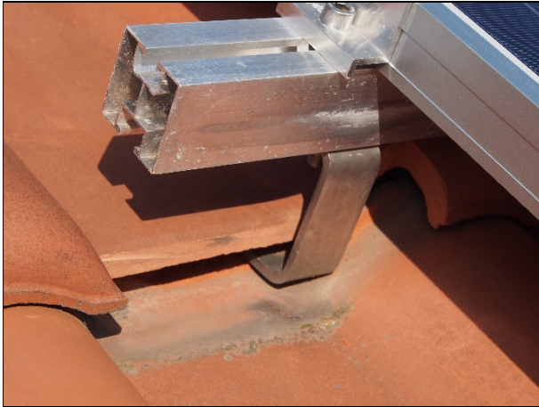
Fig. 5 The bottom rib of this tile was completely removed, which caused a great gap in the roofing layer.
