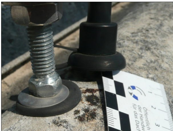
Fig. 7 Due to the new fastening installed closely to the old one, the load was removed from the fixation of the corrugated sheets with the result of leaks.
