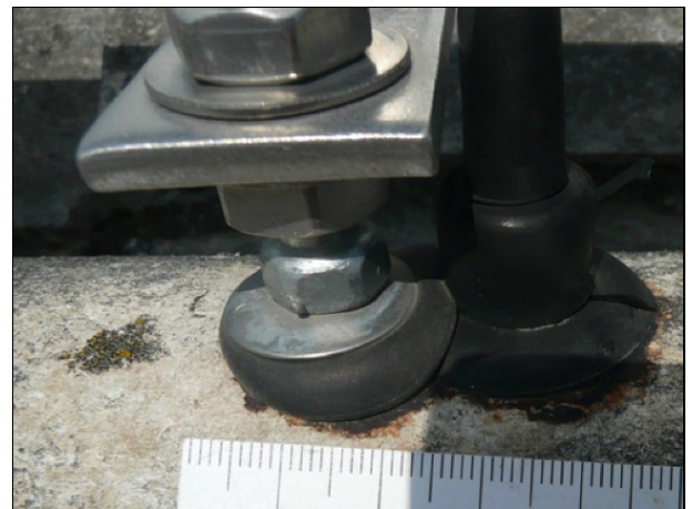
Fig. 8 Waterproofing elements placed one above the other/ screws narrowly fixed to each other led to damage and the risk of breaking
